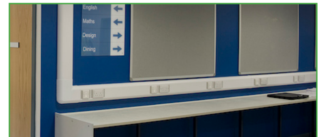
Overview of uPVC Perimeter Trunking Systems
