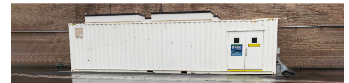
Zinc treatment system.
